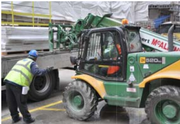
Figure 2 Off-loading a delivery from the London Construction Consolidation Centre at the Quadrant project in central London
